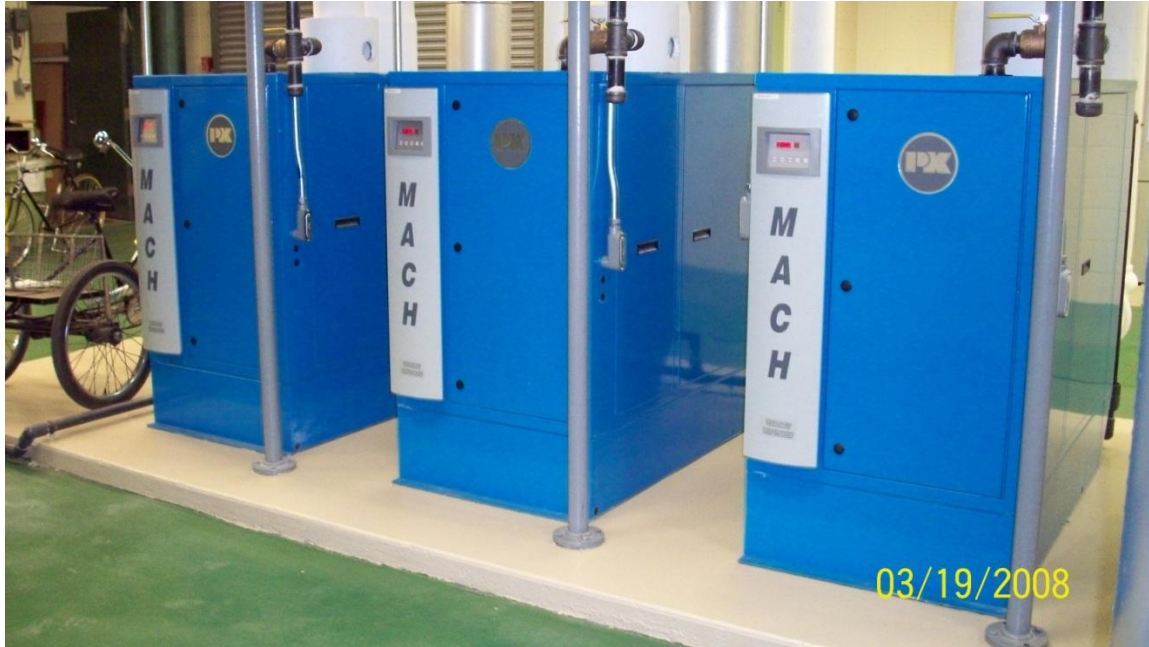
Patterson-Kelley Mach C2000's installed at Bass Pro Shops
