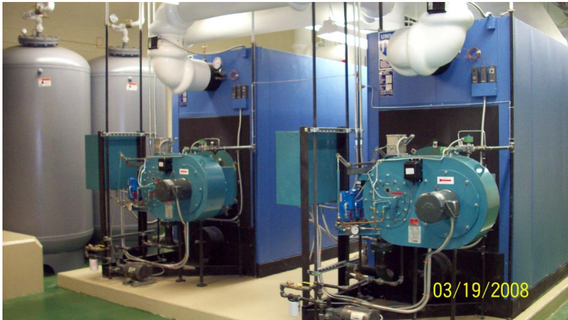
Unilux ZF1200's installed at Bass Pro Shops
